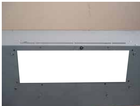
Horizontal Ducting (3-1/4"x10" Rectangular)
